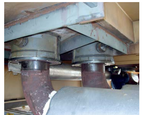
Penetration slider seal, installed on bottom of boiler.
