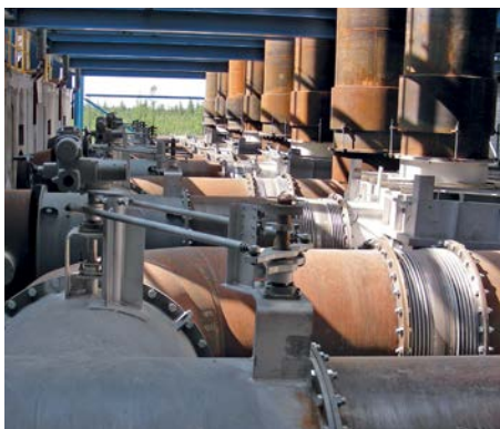
US-types installed in a flue gas system.
