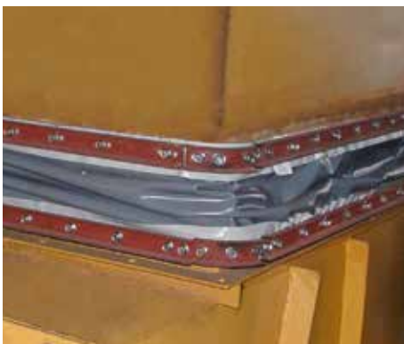
KE-Flex installed in an air duct.
