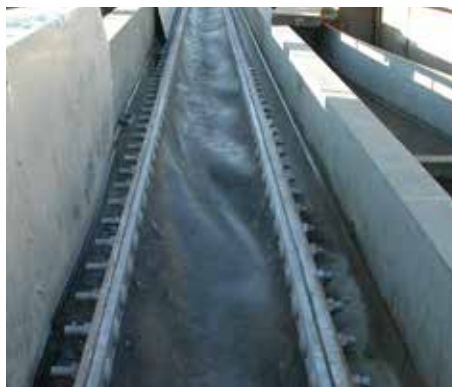
Fluachem Elastomer installed in a horizontal duct.
