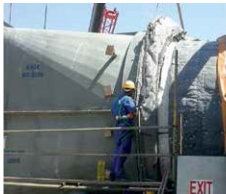
Installation of fabric expansion joint between the diffuser and diverter in a gas turbine system.
